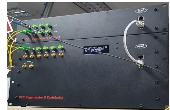
Regenerator laser station
