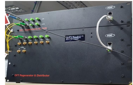
Regenerator laser station
